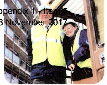
Board Members Councillor Hugh Barrett and Irene Lawrance, at the start of the Lodge Court demolition.
